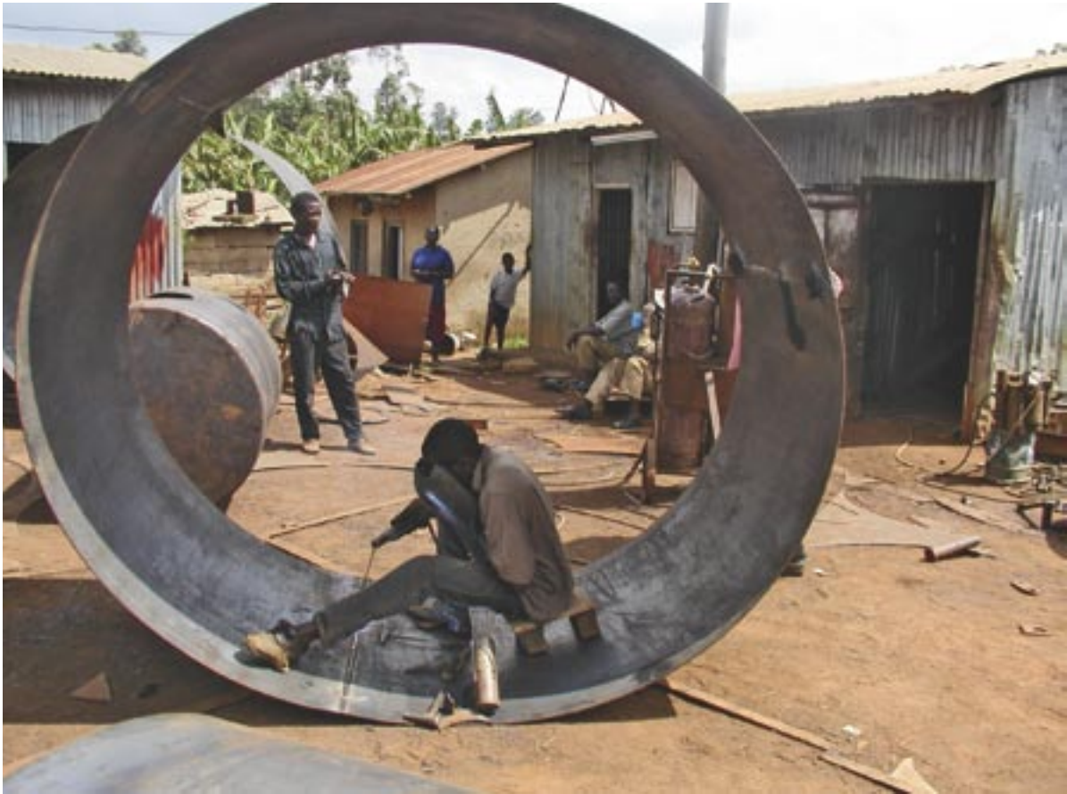
Ex-combatants manufacturing a water tank. Employing ex-combatants in short term projects advances reconstruction and community reconciliation.
